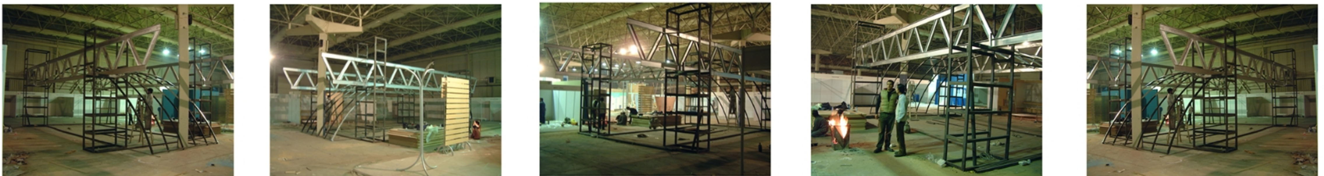
The pictures above represent the construction process at the convention center hall.
